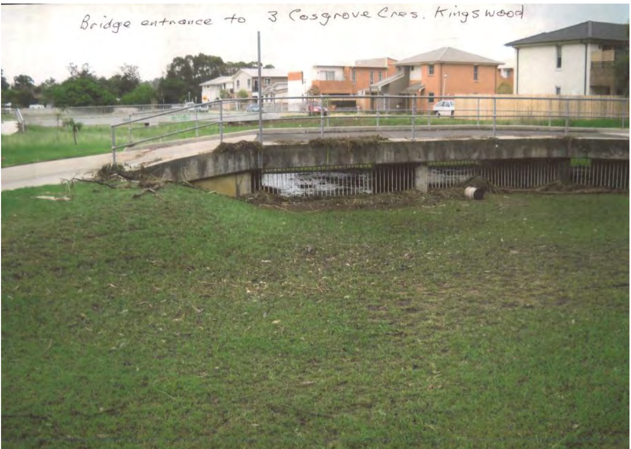
Debris marks across driveway culverts at Cosgrove Cres
