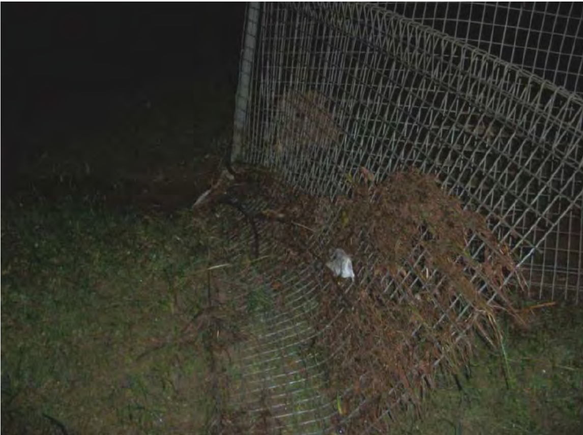
Western Sydney University Fence adjoining Second Ave showing debris mark approximately 0.5 metres high
