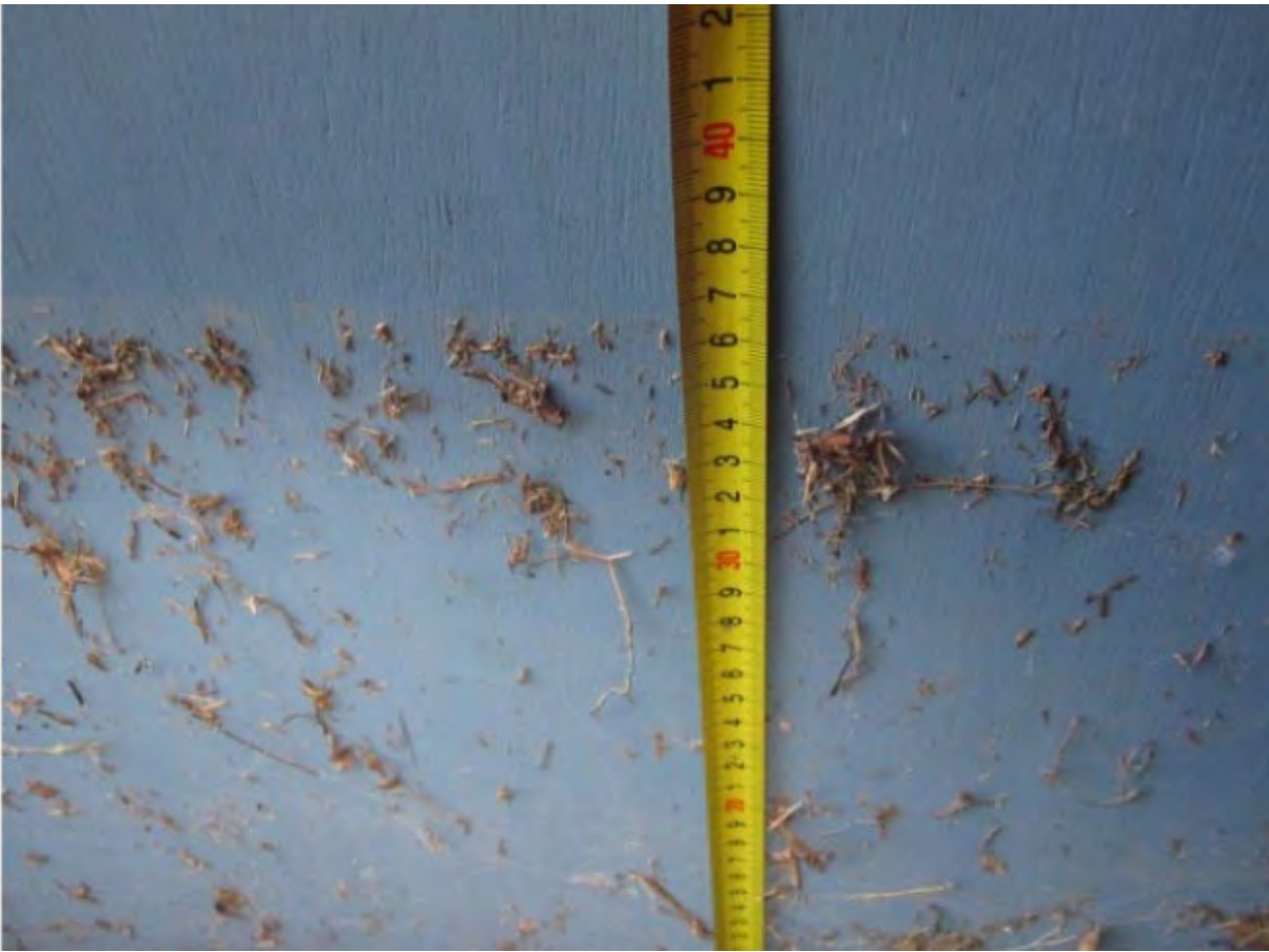
Debris mark in switch room of Kingswood Sports Club
