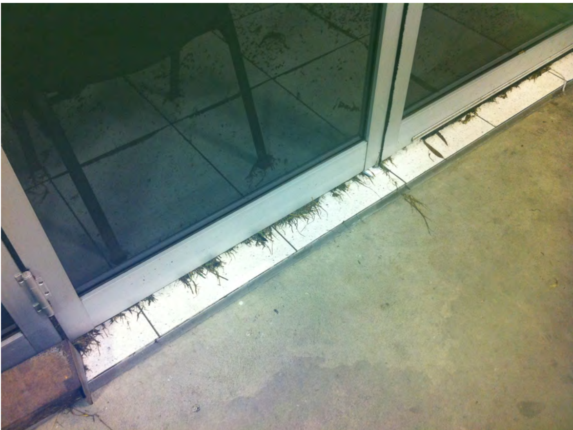
Above floor inundation at Morley Ave, Kingswood
