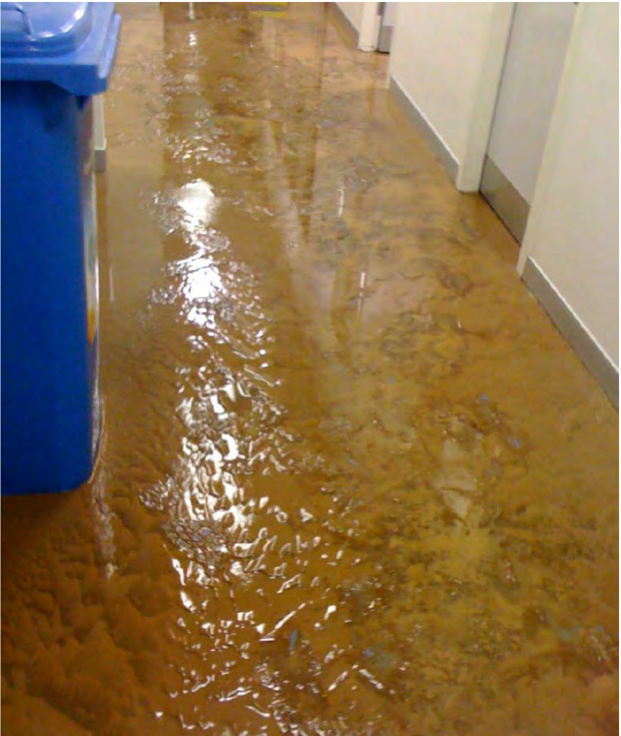
Sediment deposited across floor of Building R at Western Sydney University after above floor inundation was experienced.
