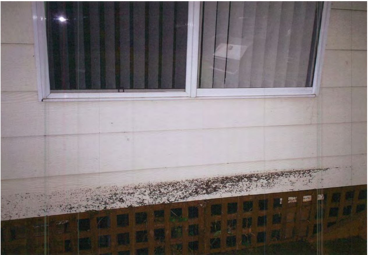
Flooding under floor at Shaw Street (estimated to be 50cm depth)
