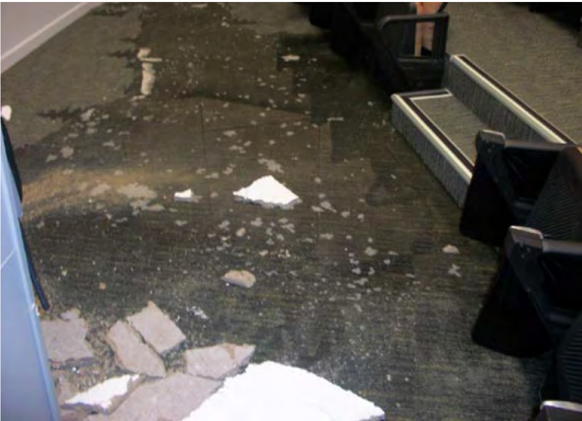
Above floor inundation at Western Sydney University
