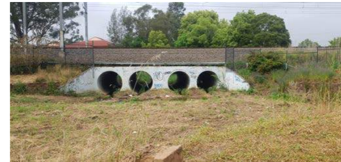
Figure 59. Existing View - Looking north at train line over drainage culverts with Great Western Highway beyond
